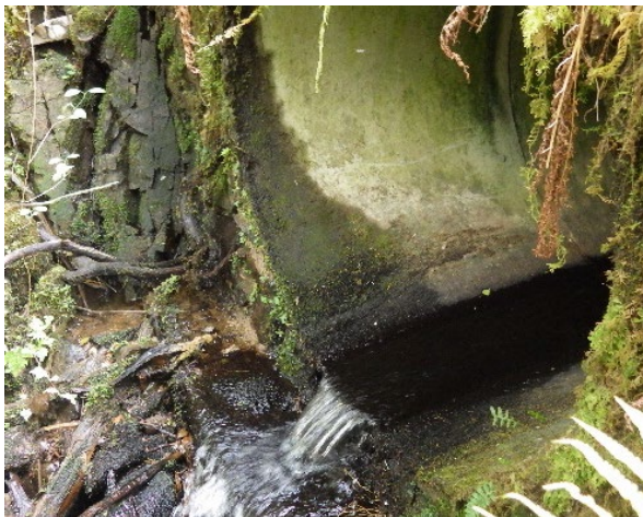
Downstream (NE) from NM 97238 31328 showing the existing culvert at the proposed crossing.
