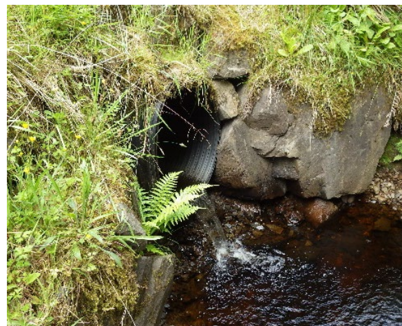
Downstream (NE) from NM 97211 30314 showing the existing culvert at the proposed crossing.
